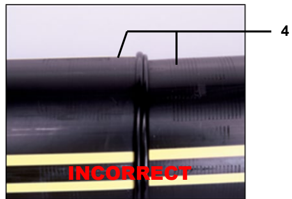
4. Improper "High-Low" alignment
